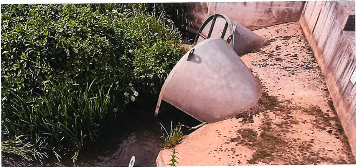
Figure 1-1. Inlet conditions on Vortex Flow Control Structure on a UK EA flood scheme (typical low flow conditions).
